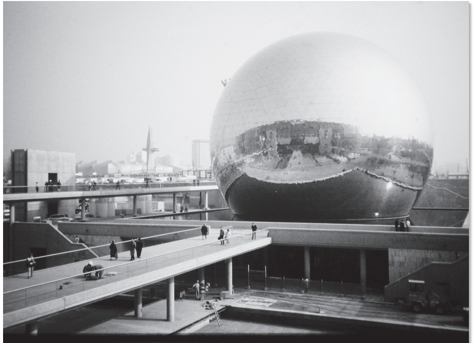
The museum under construction reflected in the just-completed outer shell of La Géode.
