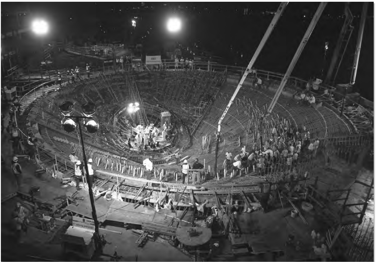
Fig. 4. View of workers and internal structure during concrete pour of the “Open Ocean” tank at the Patricia and Phillip Frost Museum of Science, scheduled to open in 2016. Courtesy of Sean Duran
